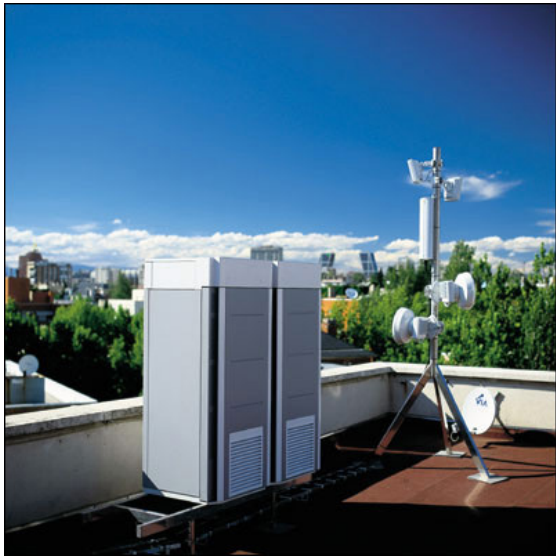
Telecom network base station
